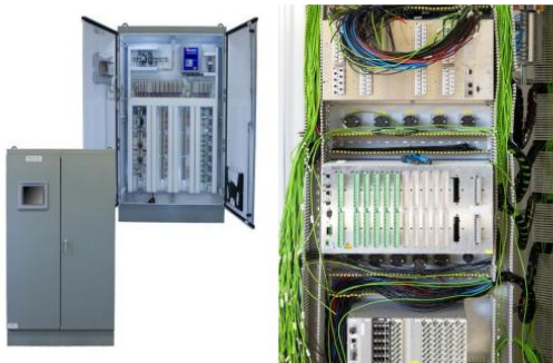
Fig 1 SCADA RTU Control Panel (Electrical Control Cabinet)
