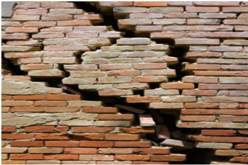
Figure – 2: Brick Work Damage
