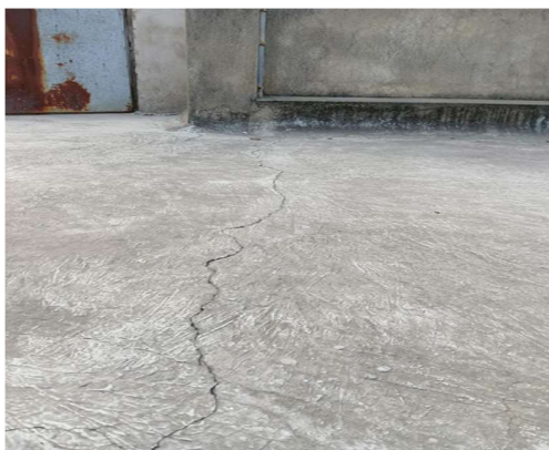
Figure – 9: Crack on roof of Old Buildings
