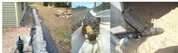
(a) French drain under construction (b) A wye-joining a perforated and solid corrugated pipe to a buried solid outlet.
