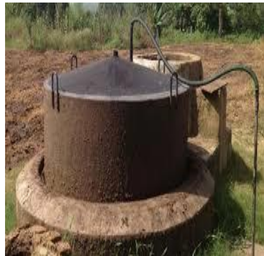
Fig.2 Floating Dome Bio gas plant
