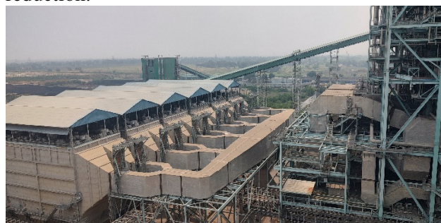
FIGURE.1.1 Boiler Duct Outer View
