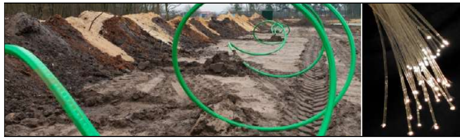
Figure 10. Cabling Pipe Lines (Left) and Silicon Fibres (Right)
