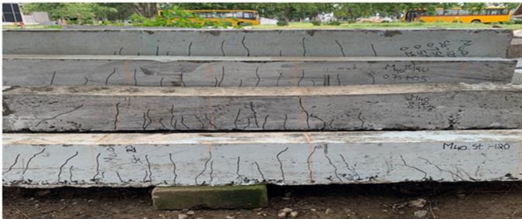
Fig. 13(b) Crack Patterns of M40 SCC Beams
